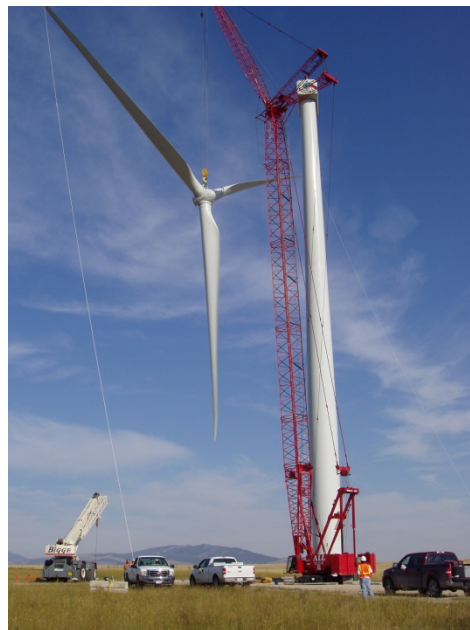
Judith Gap Energy Center - Montana
